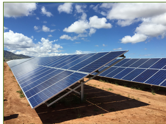
Fort Huachuca, Arizona ~18 MW solar project September 2014.
