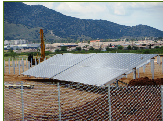
The first of ~57,000 panels emplaced at Fort Huachuca Arizona, ~18 MW project August 2014
